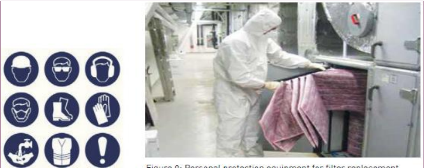
Figure 9: Personal protection equipment for filter replacement
